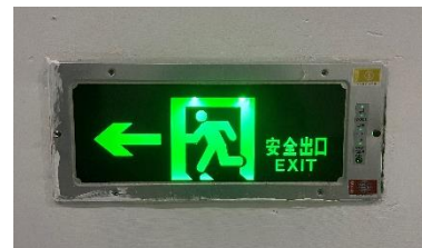
(b) Embedded safety evacuation sign
