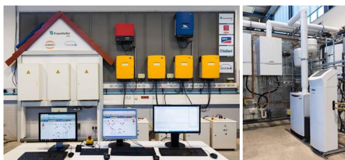
Figure 2 “Ine-Ves” test environment of a PV-CHP hybrid system. Left panel: Converters and the batteries are shown in the back. One of the computers is running the OGEMA energy management system, containing the optimizer, while the other computer holds the control unit for the entire hybrid system tests. Right panel: the gas boiler and the Vaillant ecoPOWER 1.0 are shown. The thermal storages and the pipe system representing the different heat cycles are behind the metal wall construction.
