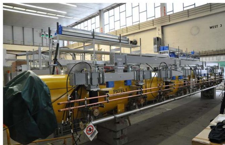
Fig. 5: Accelerator module and RF waveguide distribution
