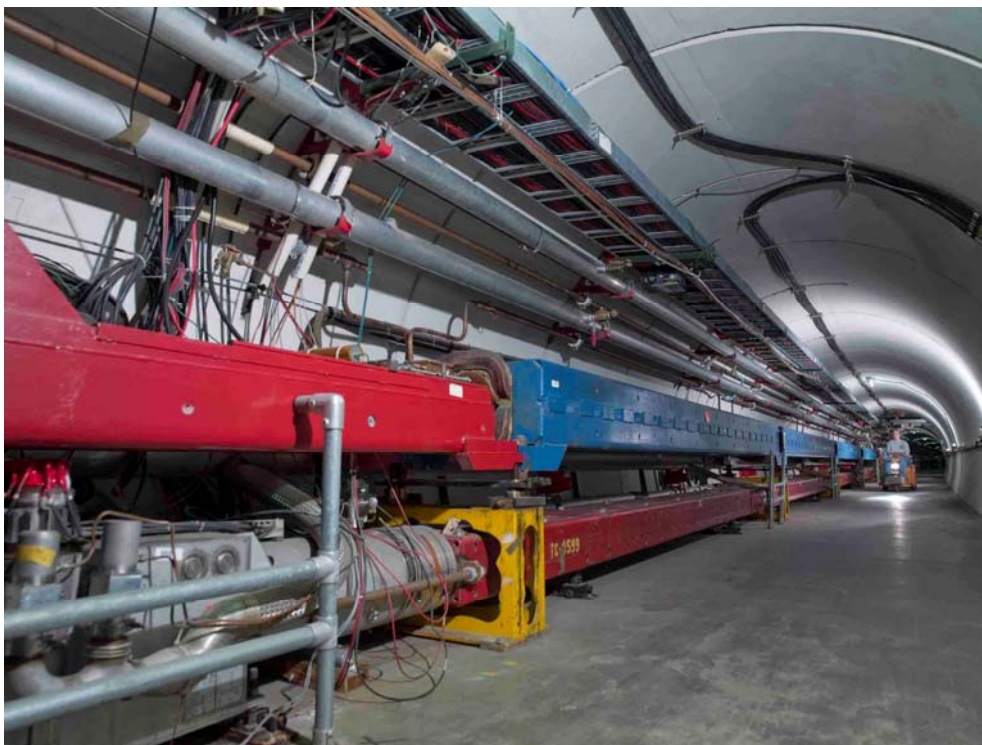
Figure 2. Superconducting magnets below the conventional magnets.
