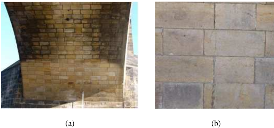
Figure 1: a) A view of a typical bridge arch showing a regular arrangement of stones in masonry, b) a crack running both across stone and along a head joint.
